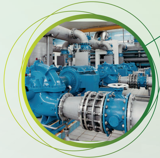
Ground Water Drainage, Riyadh.
