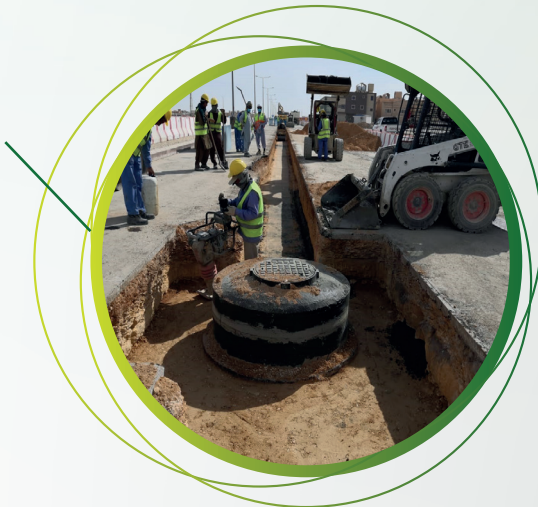
Sewer Lines, Al-Zulfi
